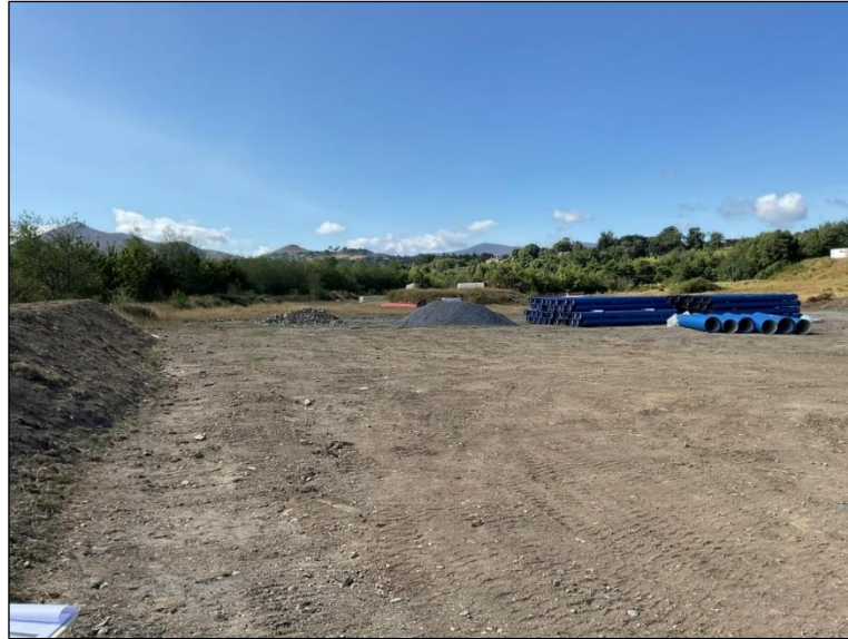
Plate 2 Stripped area on the north with rough vegetation visible to south, facing south
